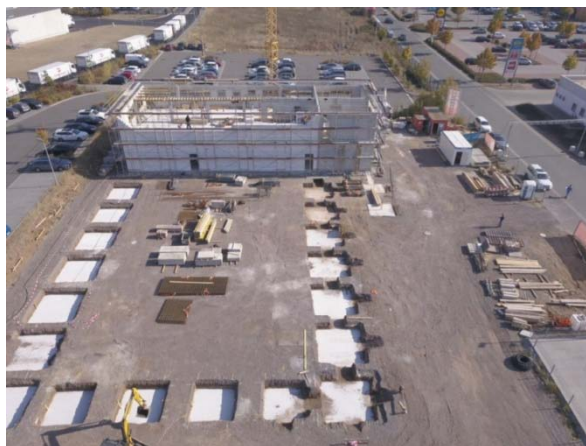
Construction project for the new office complex and the new logistics center of our subsidiary Emtron in Riedstadt
